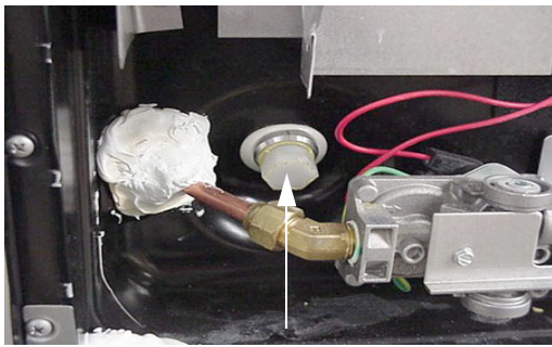
Water Heater Drain Plug (Remove with socket)
