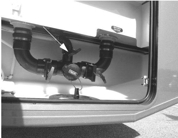
Black Waste Tank Drain Valve #2 (Front) (Located in water service center) -Typical View
