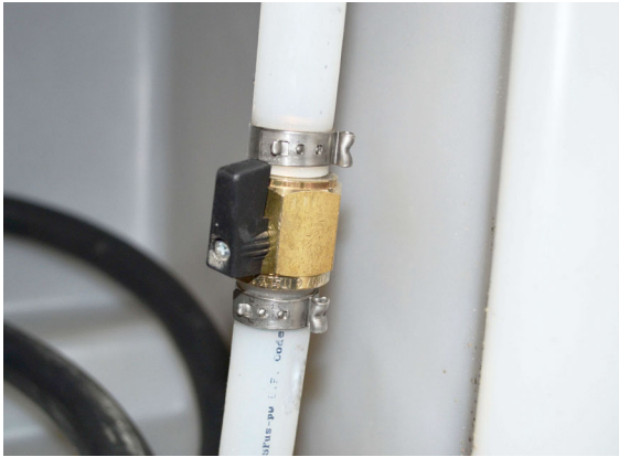
Water Tank Drain Valve -Typical installation shown
