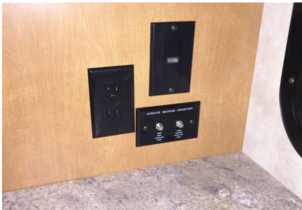
Bedroom DVD/Satellite Receiver Connection -Typical View
