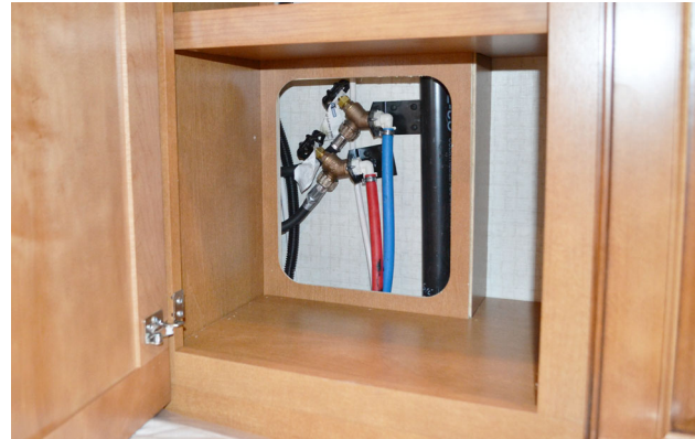
Water Supply Faucets (Located inside cabinet front of washer/dryer - remove access panel)
